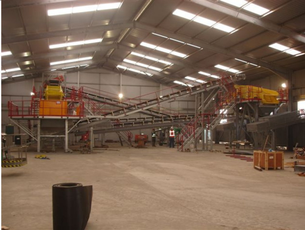
Plate 2 - IBA Processing unit inside the operational building.
